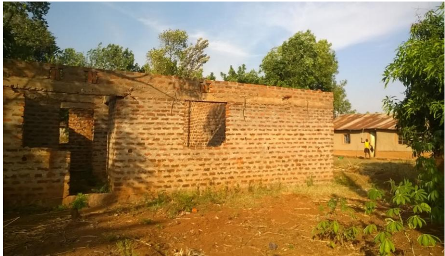
A two bedroom house being constructed by a PEEP Group member through a loan from the PEEP Group
